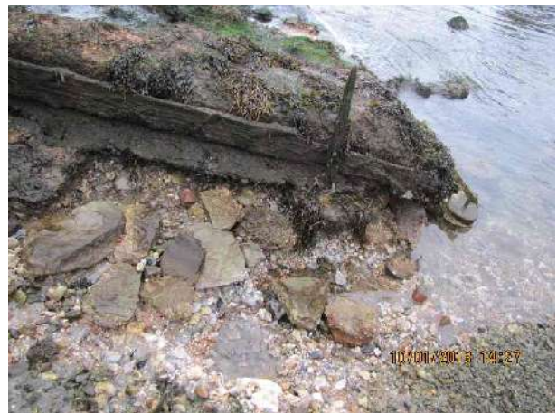
Erosion at apron
