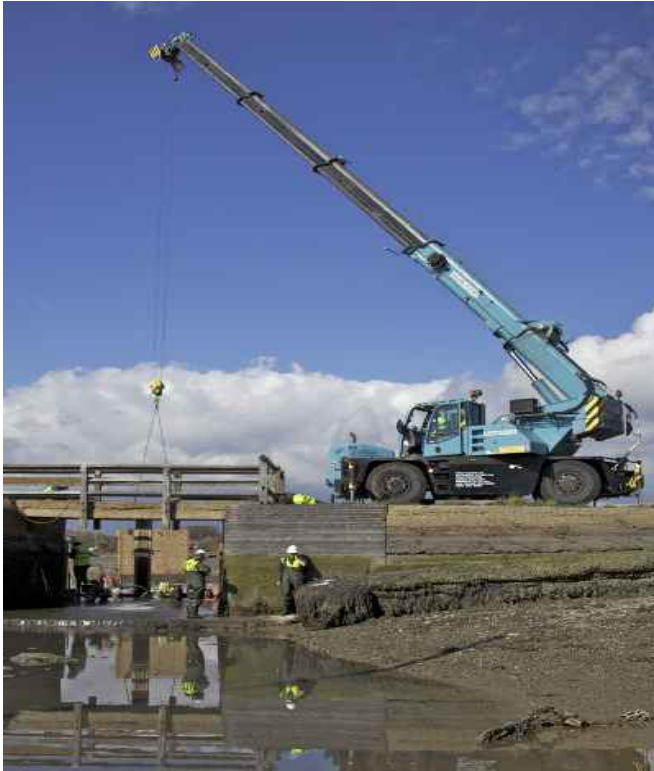
Gate being lowered Richard Somers Cocls
