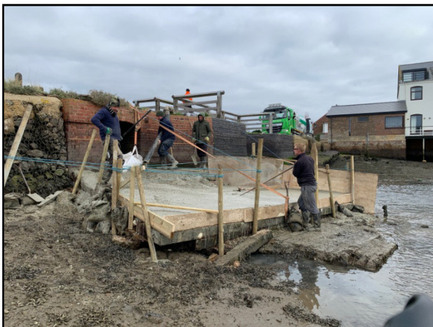
IN PROGRESS – Sluice Apron viewed from the south showing lorry delivering concrete
