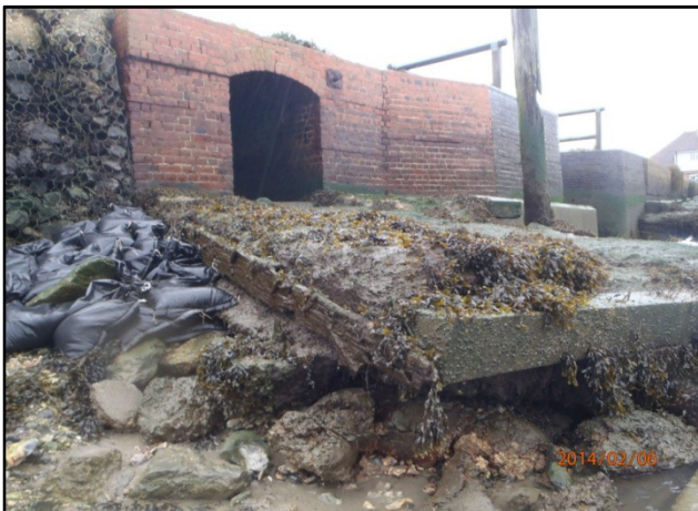
BEFORE - Damaged Sluice Apron viewed from the south showing rotten post to be removed
