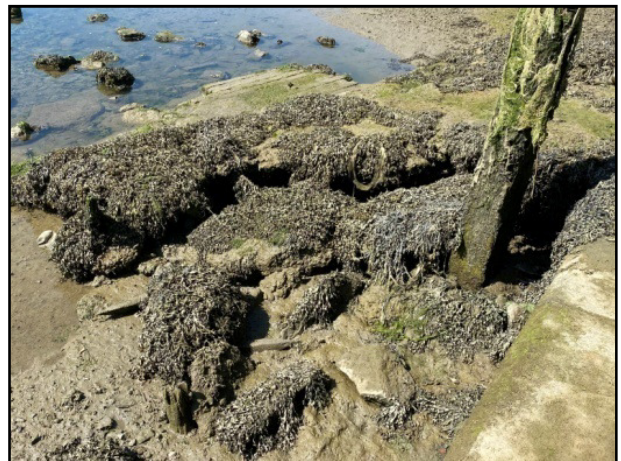
BEFORE - Damaged Sluice Apron viewed from footbridge
