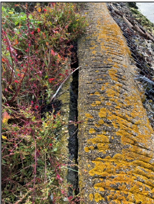
Crack along south-west corner
