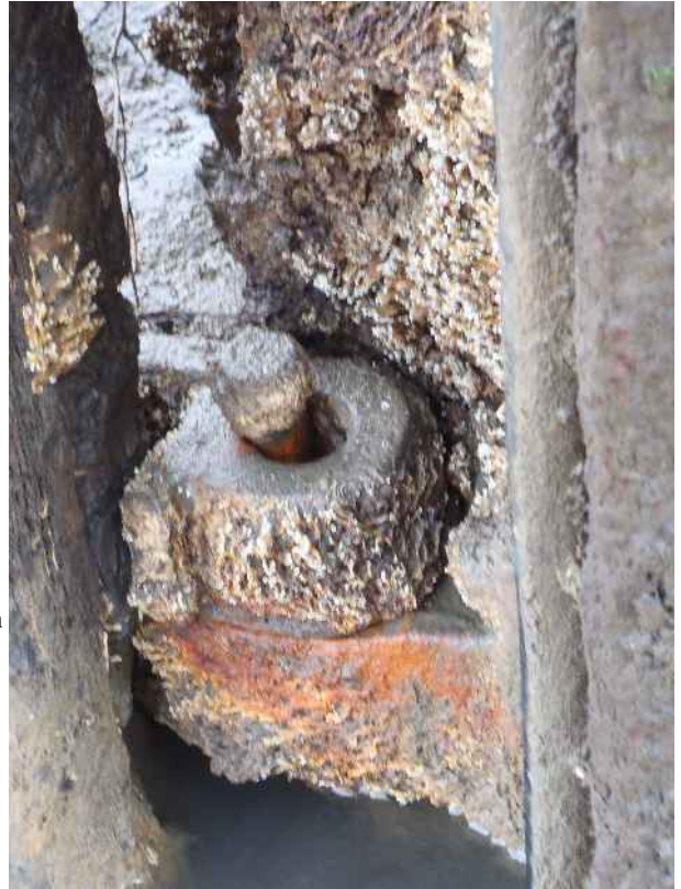
Lower hinge with worn pintle - to be replaced
