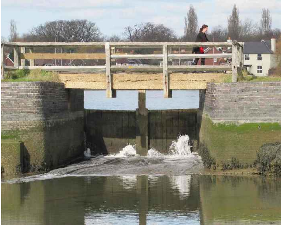
Pond gates leaking
